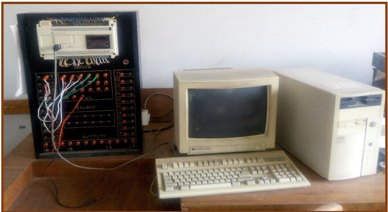
Programmable logic controller board 2
